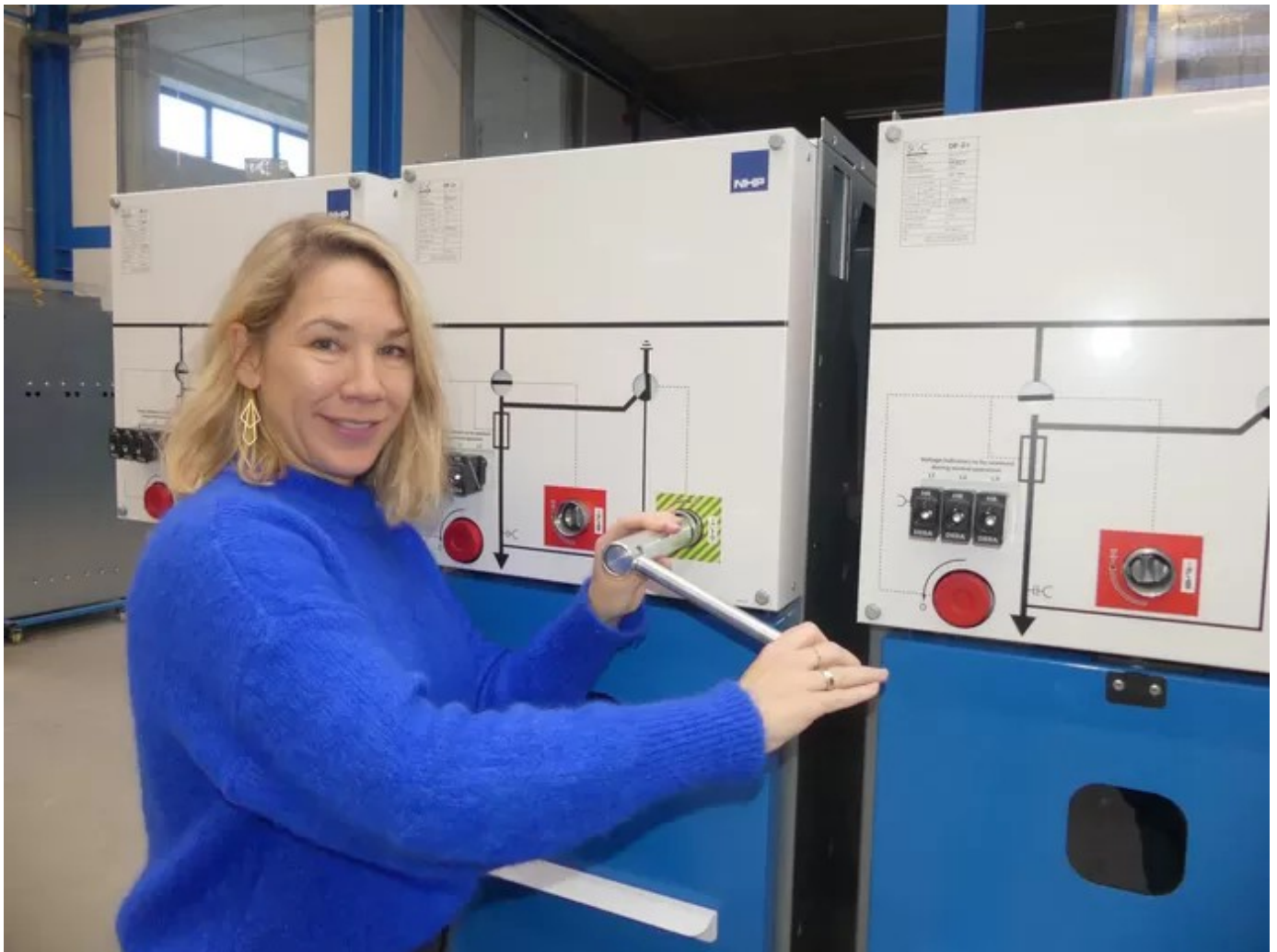
Sophie Vandoorne at the cubicles of her company SwitchGear Company. © Anthony Stadius
