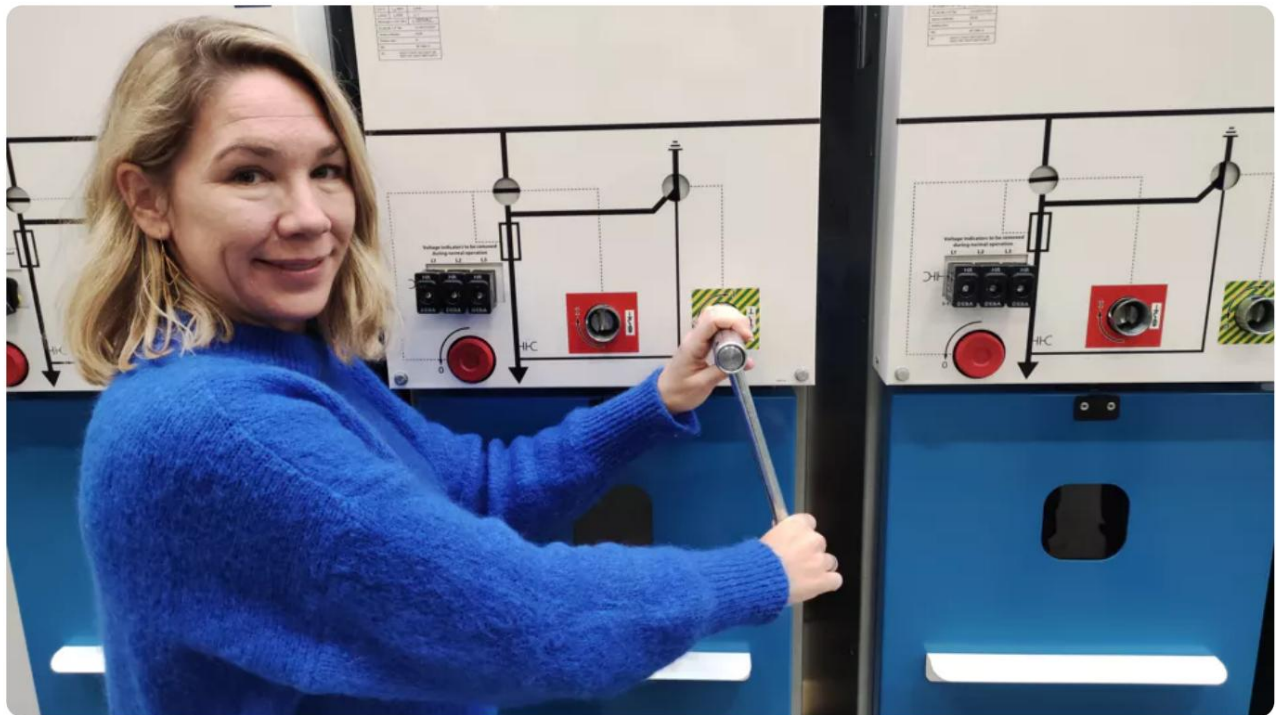
Sophie Vandoorne at a switch box that supplies the antennas with power
